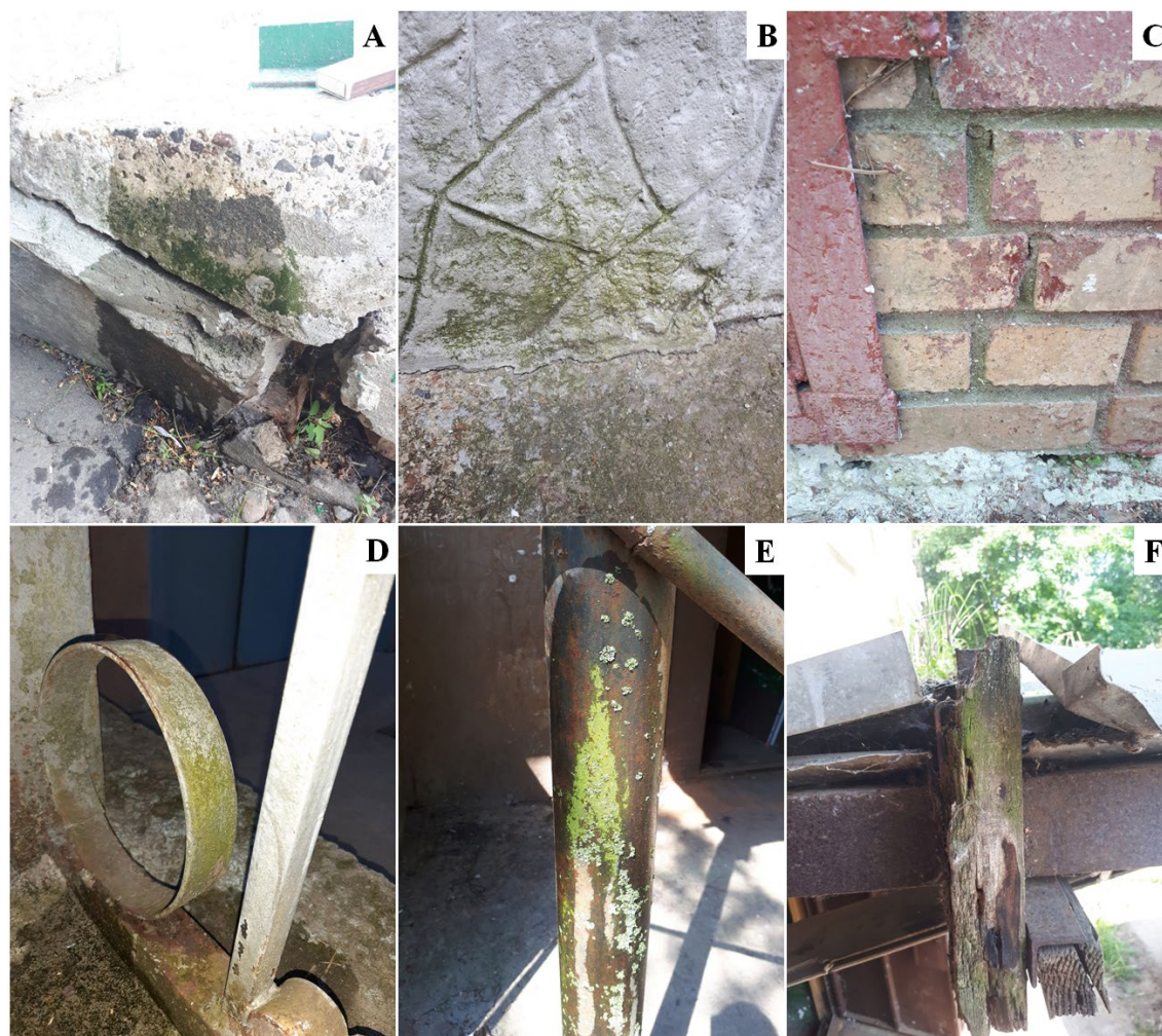
Fig.1. Sampling sites for biofilms. A – entrance steps; B – plastered basement of a residential building; C – brick wall, mortar joint; D – bottom of the metal canopy support; E – metal canopy support; F – wooden canopy support.
